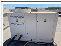
#9: Air Conditioning, Boiler and mixer Unit
