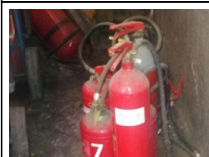
#10: Fire Extinguishers and First Aid Boxes
