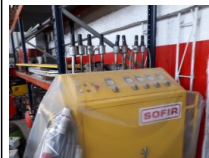
#24: Electric Control Unit
