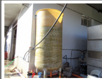
#1: N. 3 Tanks and Hydraulic Pump
